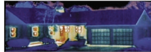
IR imaging shows heat escaping from a house during those expensive winter heating months.
